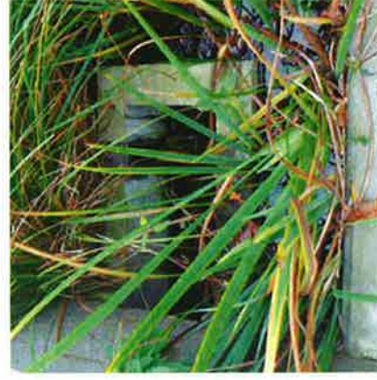
Example of a notched overflow
