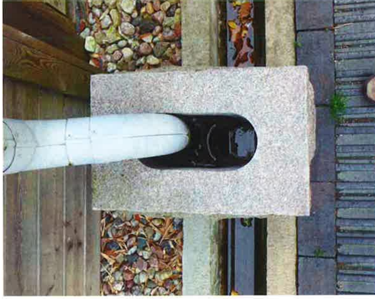
Down pipe empties to rill Malmo, Sweden
